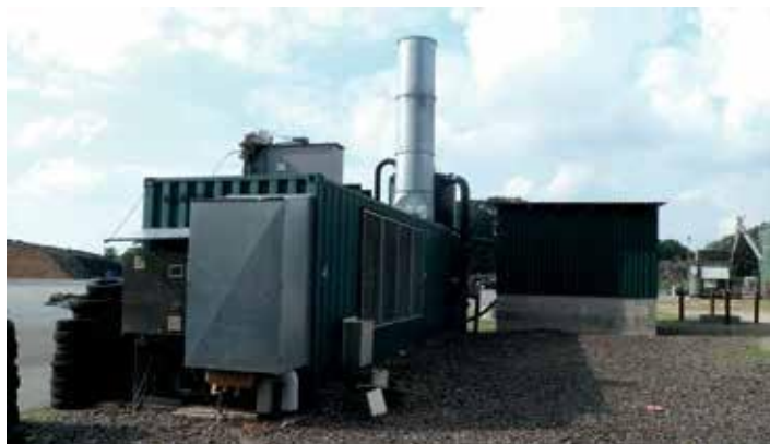
Figure 1. The containerised dryer. The front metal box contains the fore- and back-run pipes of the CHP. Behind the stack on top of the container: the buffer tank for raw digestate
