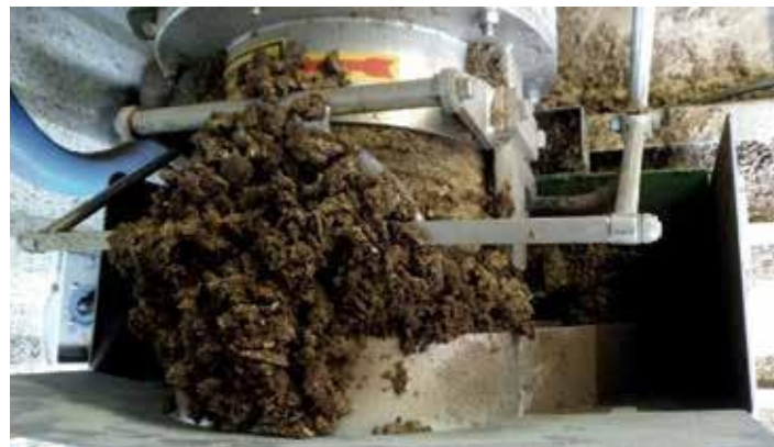
Figure 3. Solid digestate from behind the dewatering with a screw press separator. This falls onto the conveyor belt of the disputable dryer
