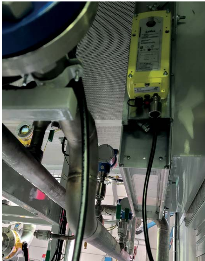
Actuator for ventilation system
