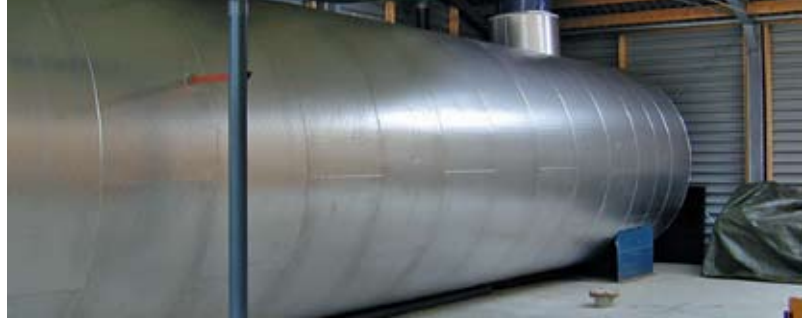
Horizontal / Plug flow digester
